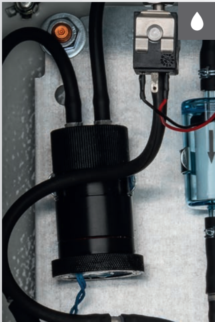
Thermal condensate monitoring for safe operation
